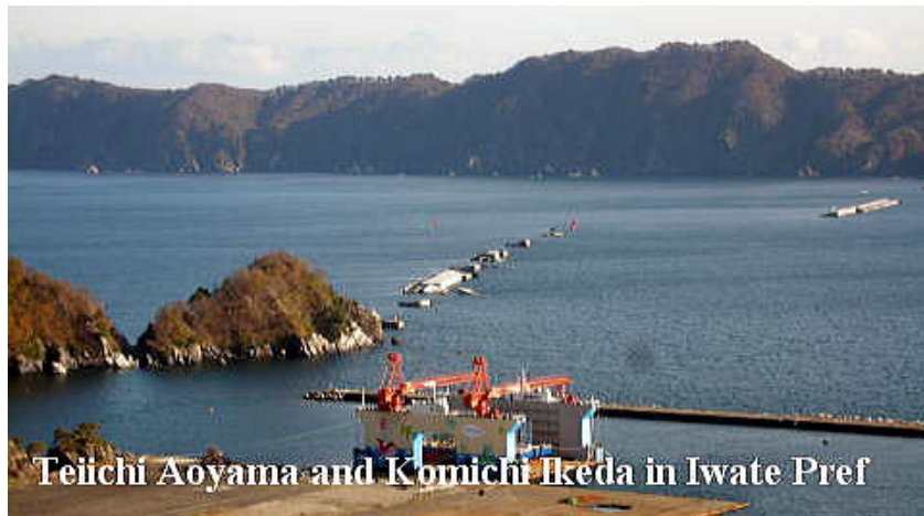
Fig.5. The breakwater at the entrance of Kamaishi bay destroyed by the tsunami (Construction cost: 120 billion yen)
