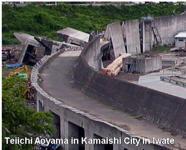
Fig.6. The tide embankment at Kojirahama fishing port in Touni Town, Kamaishi city, destroyed by the tsunami
